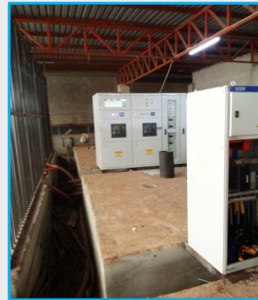
Industrial and domestic Electrical Installation
